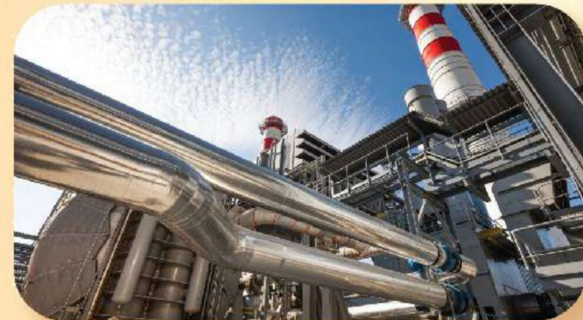
THERMAL POWER STATION
